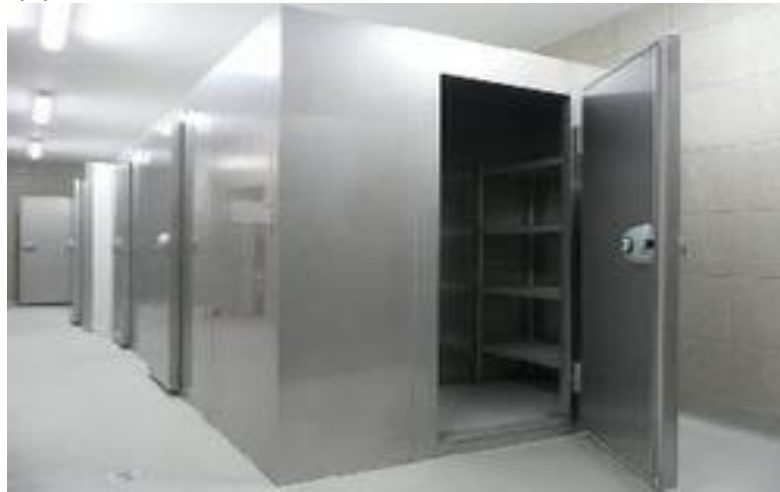
(E) COLD ROOM
