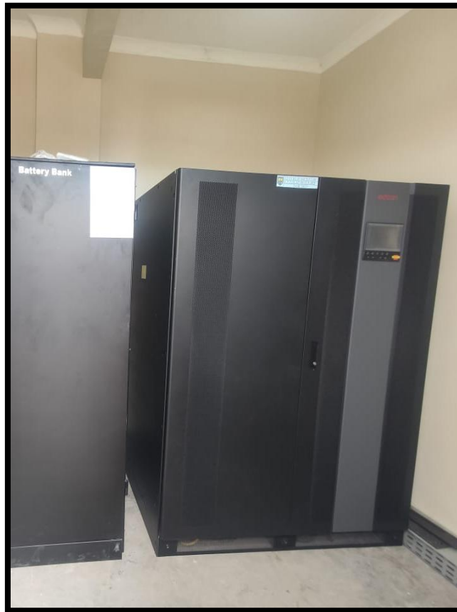
Gambar 21 Sarana Prasarana Genset Mesin UPS
